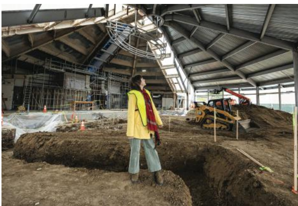
PICTURED ABOVE: Madison Zuniga in the CU Center construction zone Photos courtesy of: Ann Ashmon
