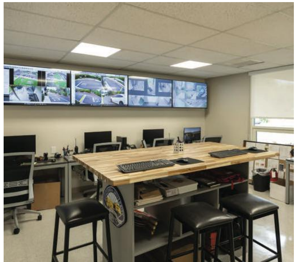
PICTURED ABOVE: Campus Safety’s new base of operations Photos courtesy of: Ann Ashmon
